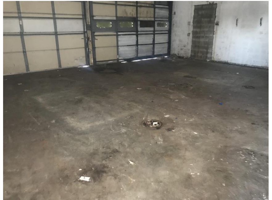
Photo 8 – A view of the interior of the service bay and floor drain.
