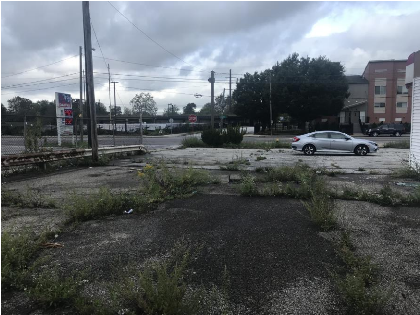
Photo 7 – A view of the parking area looking west towards Euclid Avenue, the solar array and residential townhomes.
